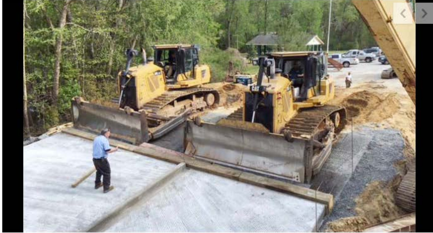
Two bulldozers push an 80-foot concrete boat ramp into Lynchies River at Venters Landing on Friday afternoon.
